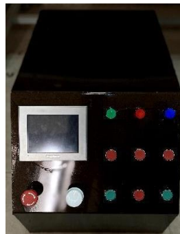
Figure 10. Control Panel of Push Buttons
